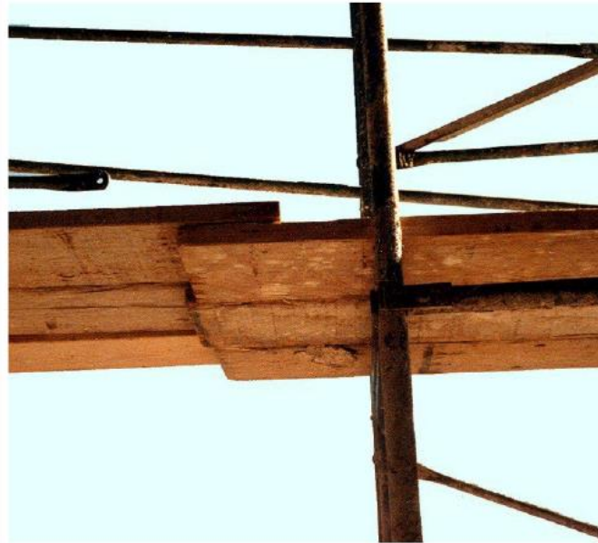
Figure 8-7 Planks Not Properly Overlapped or Supported
