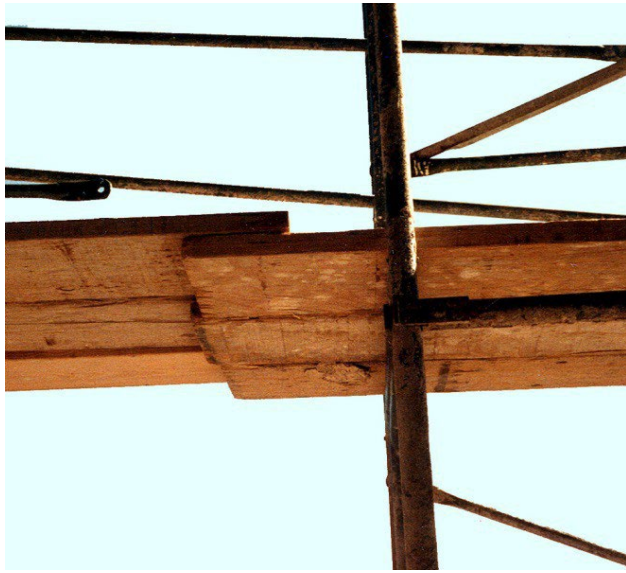
Figure 8-7 Planks Not Properly Overlapped or Supported
