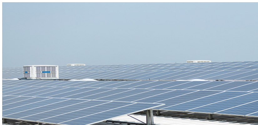
Figure 5: Rooftop Solar Panels
