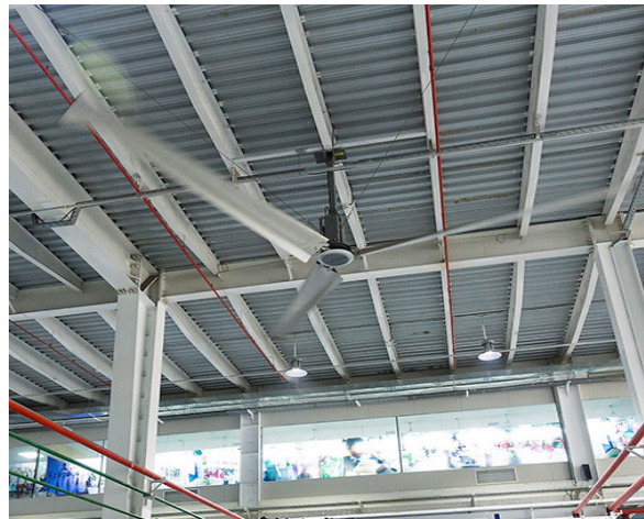
Figure 4: HVLS Fans in the Sewing Area
