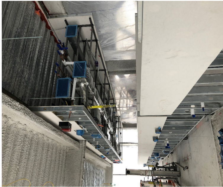
Figure 7: Installed MEP Rack System
